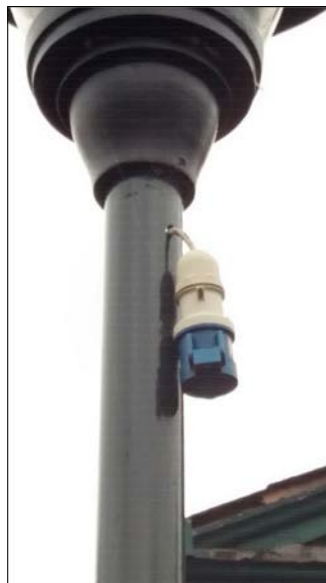
Figure 11.2 - Unacceptable cable entry in column – provide grommet and affix the socket to the column
