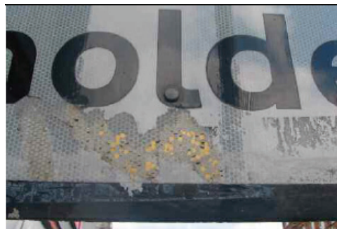
Removal of graffiti can damage the retroreflective surface of signs
