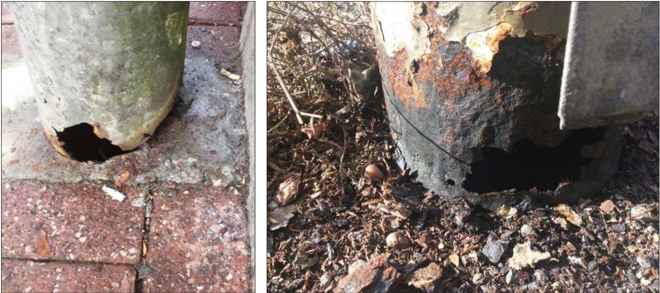
Pictures A12.23 and A12.24: Above ground corrosion
