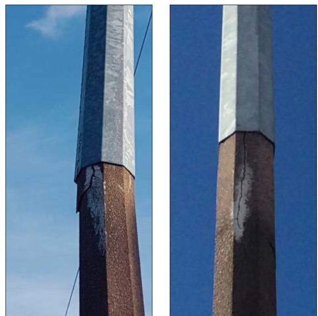
Pictures A12.12 and A12.13: Cracking of column shaft below the sleeve bracket
