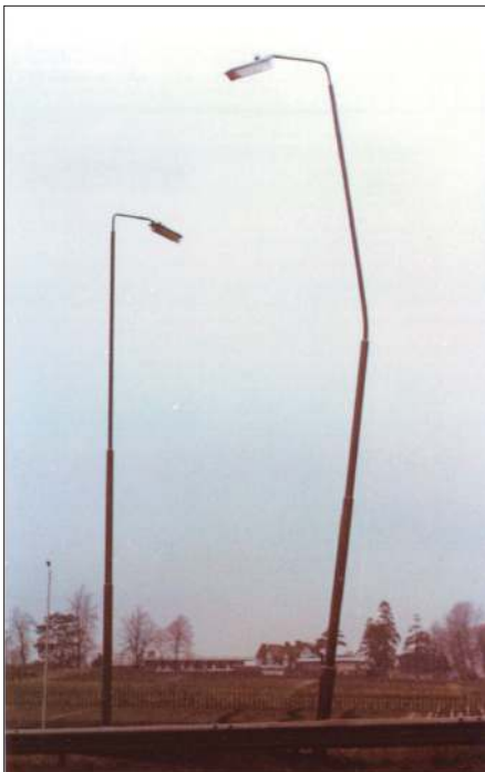
Picture A12.31; Severe column distortion caused by impact damage
