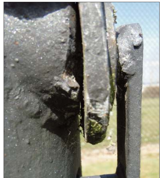
Picture A12.33: Corrosion and cracking at hinge support
