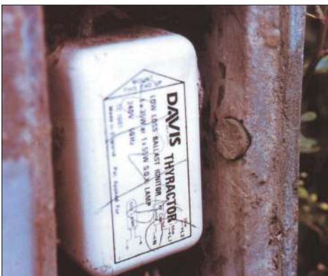
Picture A12.17: Potential failure at spacing plugs inside the door opening of a concrete lighting column
