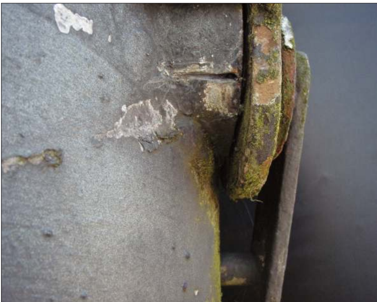
Picture A12.32: Cracking at hinge support
