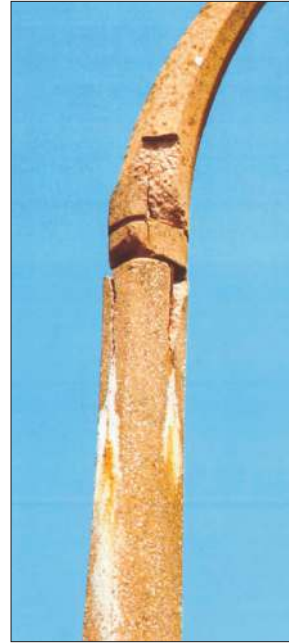
Picture A12.18: Deterioration at a concrete column bracket joint aggravated by lack of sealing or maintenance of sealing during column life.
