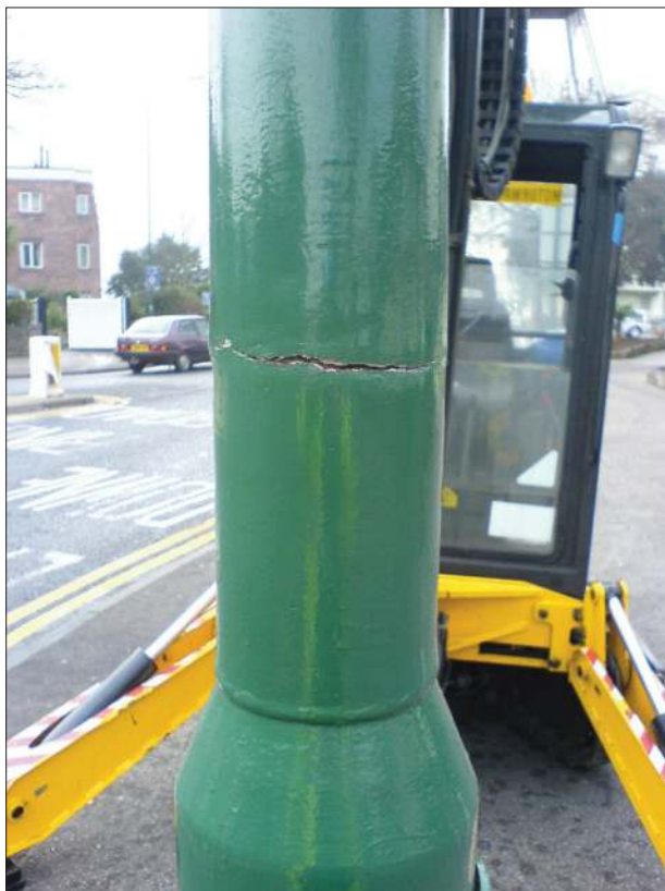
Picture A12.27: Internal corrosion from swage joint
