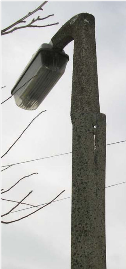
Picture A12.14: Cracking at bracket/shaft joint
