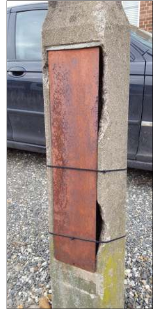
Picture A12.19: Damage around the door opening on a concrete column which could eventually result in exposure and corrosion of the embedded reinforcement.
