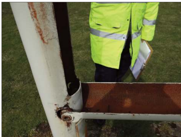
Picture A12.34: Corrosion at hinge support
