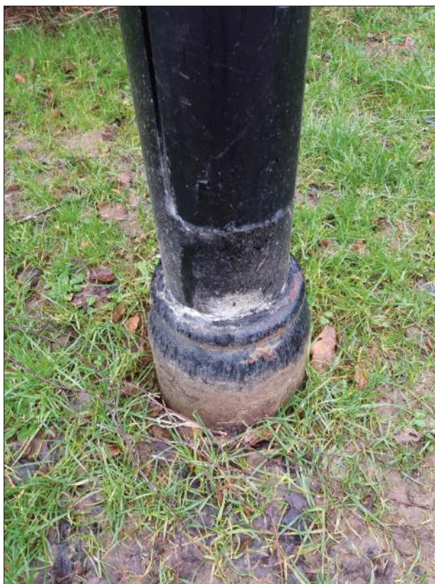
Picture A12.22: Early onset of corrosion caused by dog urine
