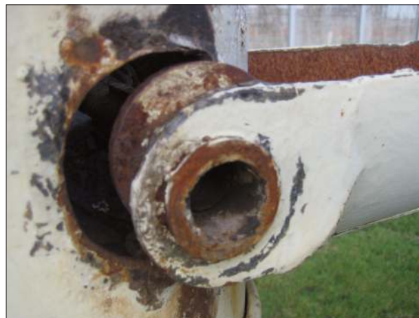
Picture A12.35: Failed hinge joint
