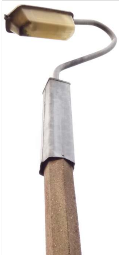
Picture A12.15: Poor fitting sleeve bracket 5m column
