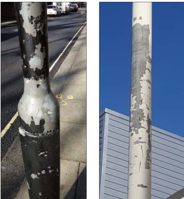
Pictures A13.1 and A13.2: Debonding of paint due to poor surface preparation
