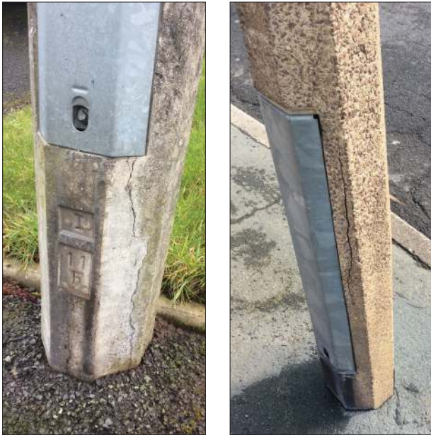
Pictures A12.10 and A12.11: Hairline cracking of concrete columns
