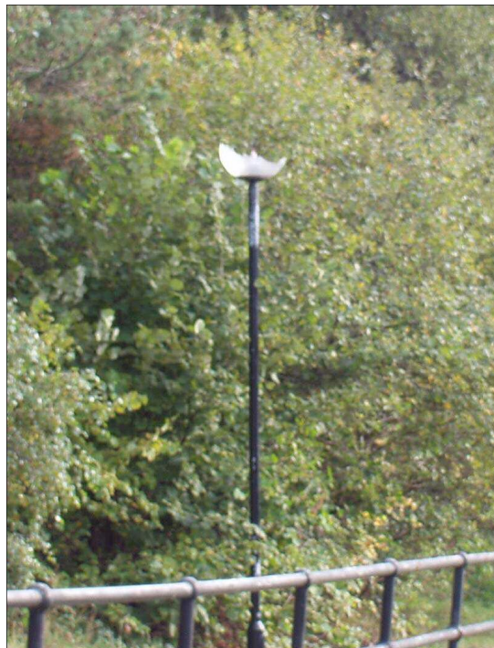
Figure 5.2 – Example of a poorly maintained Lighting Column
