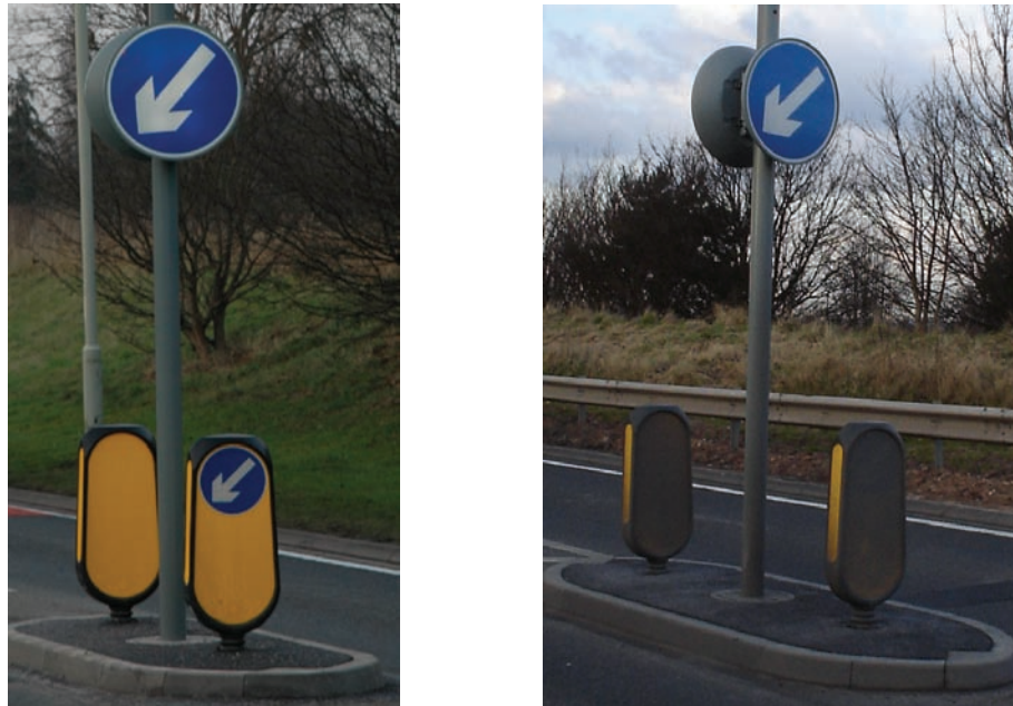
Figure 19 – Retroreflective bollards shown when newly installed (left) and less than a month later (right), at the same location (Photos courtesy of Simmonsigns Ltd)
