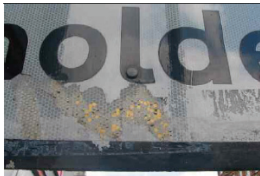
Figure 12 – Removal of graffiti can damage the retroreflective surface of signs
